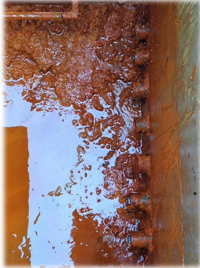
Photograph 16 – Horizontal outlet drain pipes at North Valley Park. Only two of the seven pipes were discharging water on March 5, 2024.
