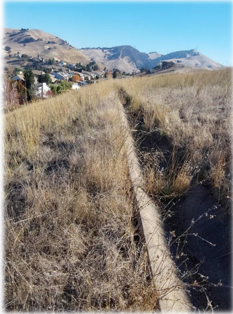
Photograph 15 – Similar conditions observed in the area as noted in March 9, 2023 letter, Photo K: separation of soil from the downhill side of the V-ditch due to slope creep.
