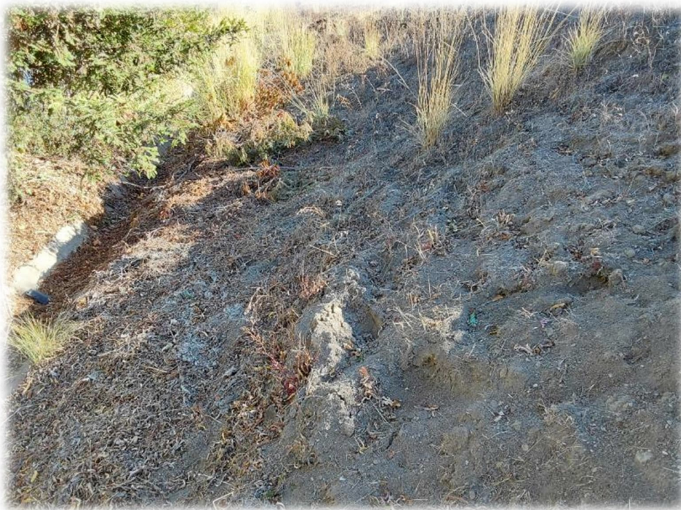
Photograph 13 – Some slope erosion/creep behind 5229 Keller Ridge Drive along with debris within V-ditch. Additional V-ditch cleaning should be performed.
