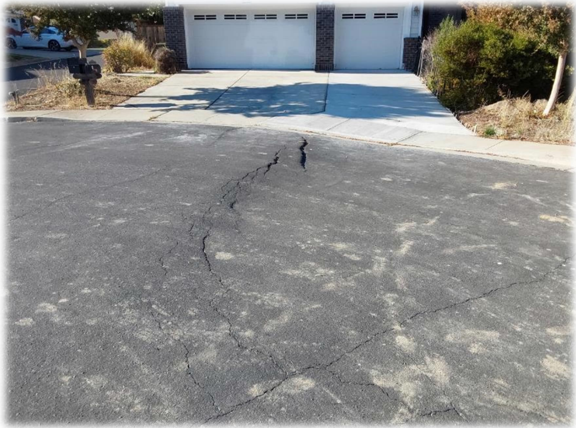
Photograph 5 – Current conditions at 8053 Kelok Way. The cracks have expanded a little and concrete in the driveway/sidewalk has been repaired since we last visited this location (see Photograph 6 below).
