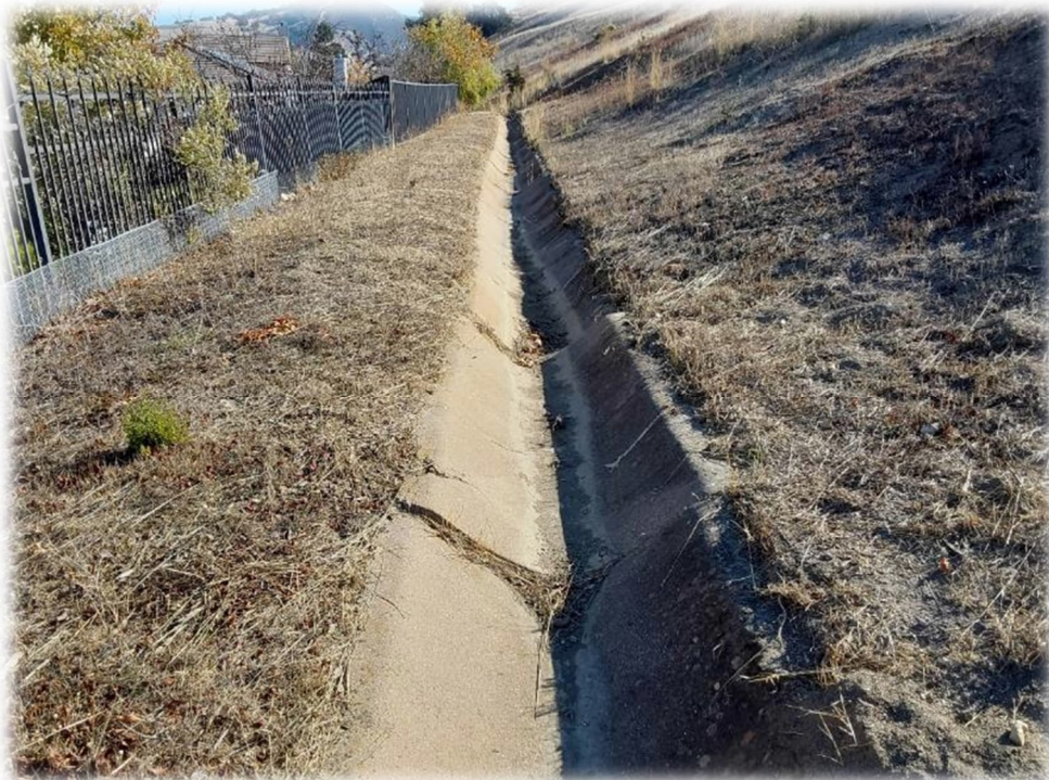
Photograph 10 – ditch condition remains similar as Photo I noted in March 9, 2023 letter: cracked and offset. V-ditch repairs should be performed.
