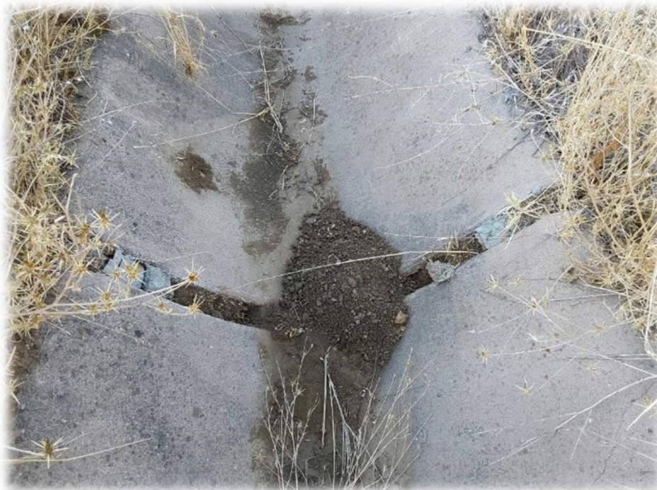
Photograph 20 – V-ditch separated at joint in the area of Photo 19. V-ditch should be repaired.
