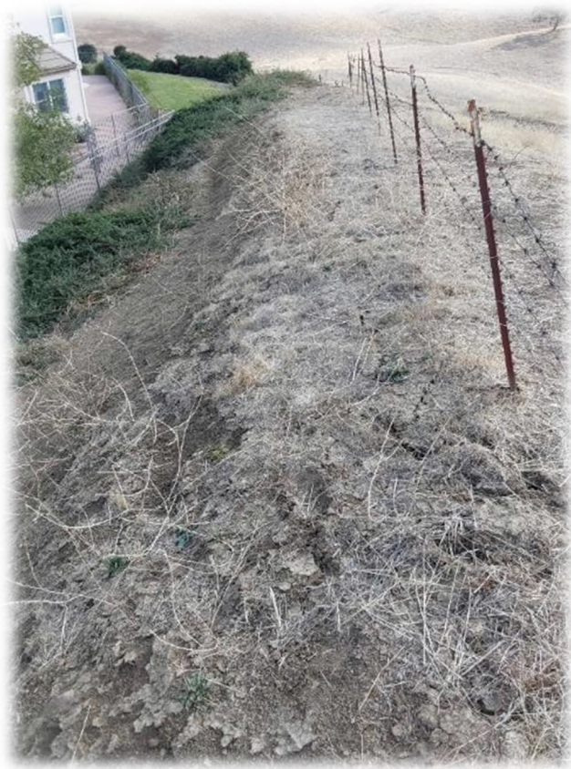
Photograph 27 – Possible slope creep/shrinkage cracks along top of slope south of 185 Brandywine Place.
