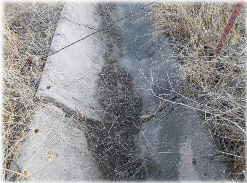
Photograph 21 – V-ditch separated at joint in the area of Photo 18. V-ditch should be repaired.
