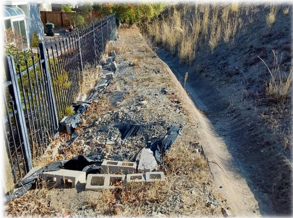
Photograph 12 – Similar conditions observed as noted in March 9, 2023 letter, Photo G: Slope creep depositing debris in V-ditch and resulting in minor cracking of V-ditch. Additional V-ditch cleaning and repairs should be performed.
