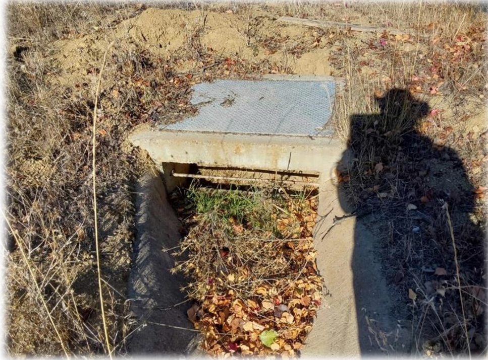
Photograph 9 – Condition of this inlet remains similar to that noted in Photo J of our March 9, 2023 letter: filled with soil/debris. Located west of 8049 Kelok Way. Additional cleaning of this inlet should be performed.
