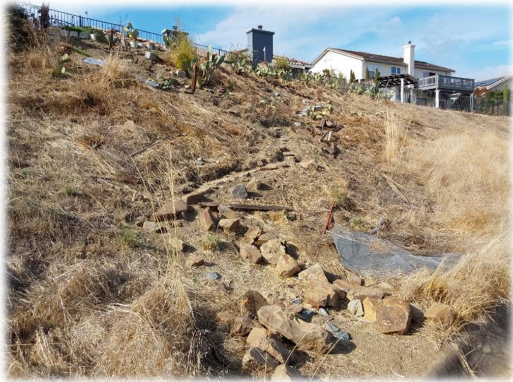
Photograph 28 – Resident at 183 Brandywine Place has added boulders and vegetation to the slope along with creating a pathway, possibly for landscaping purposes. It is not an ideal situation to regrade the slope.
