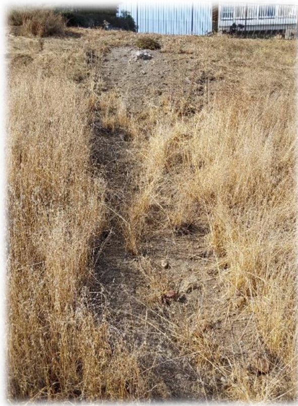
Photograph 30 – Minor slope wash along slope at 179 Brandywine Place.
