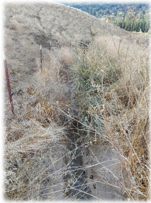
Photograph 18 – Additional cleaning of V-ditches along the slope should be performed.
