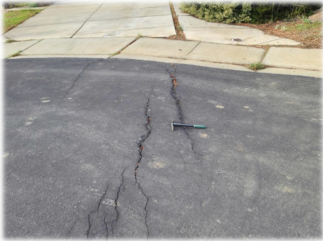
Photograph 6 – Previous conditions at 8053 Kelok Way on December 8, 2022.
