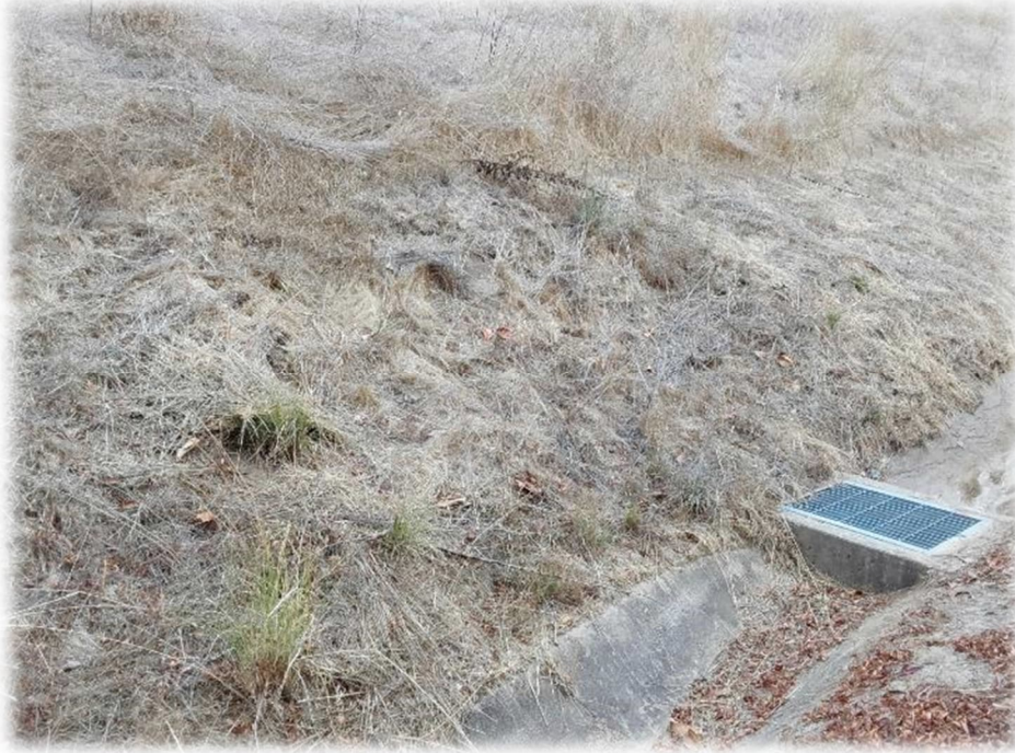
Photograph 3 – Shallow raveling/settlement above a drop inlet uphill from 3053/3055 Windmill Canyon Drive. Condition remains the same as observed in early 2023 (see Photo B in letter dated March 9, 2023). There is a pipe coming downhill into inlet, likely from upper V-ditch. Possibly, this area experienced some settlement.
