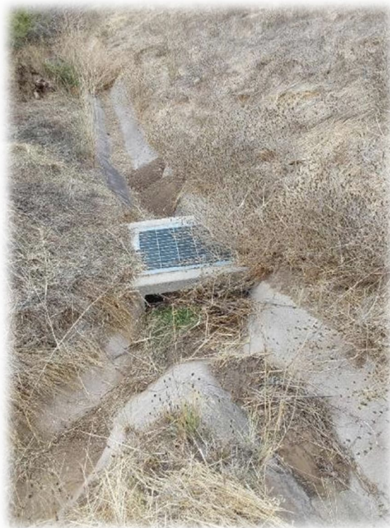
Photograph 2 – V-ditch filled with soil and vegetation behind 3041 Windmill Canyon Drive. Throughout this area, V-ditches contain soil and debris originating from burrowing animal activity, vegetation, etc. Additional V-ditch cleaning should be performed.
