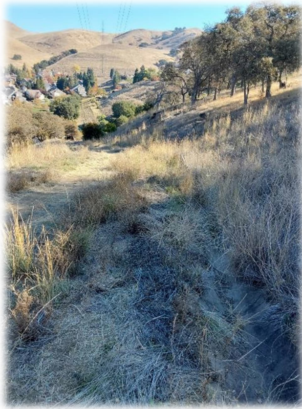
Photograph 7 – V-ditches located along the slope north of Kelok Way contain debris and cracking. Additional V-ditch cleaning and repairs should be performed.
