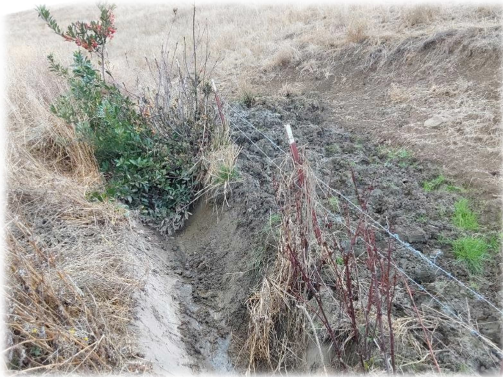
Photograph 19 – Similar conditions as noted in March 9, 2023 letter, Photo O: slope creep and minor sloughing adjacent to V-ditch.
