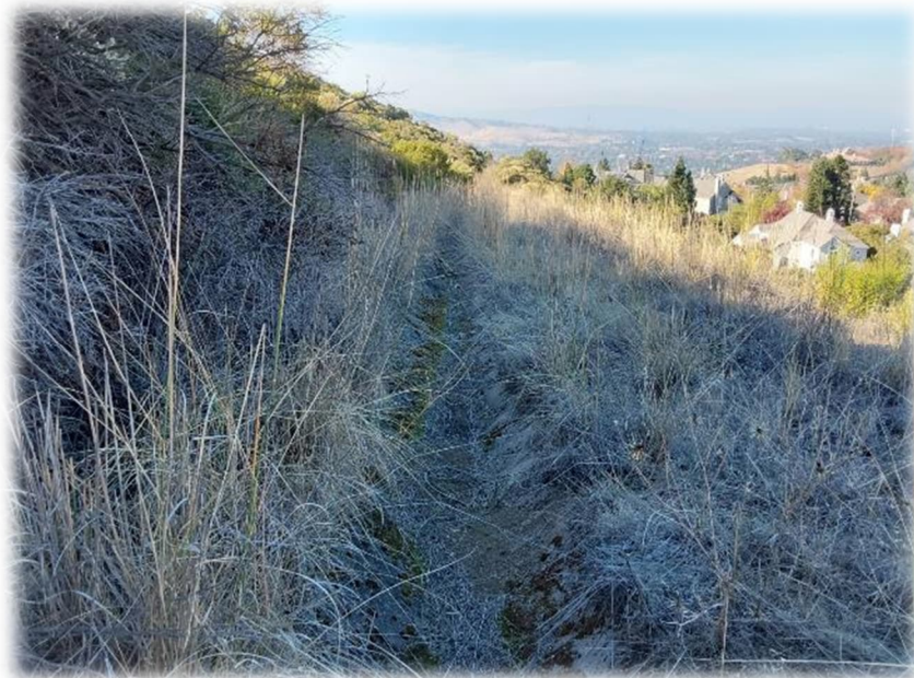
Photograph 8 – V-ditches located along the slope north of Kelok Way contain debris and cracking. Additional V-ditch cleaning and repairs should be performed.
