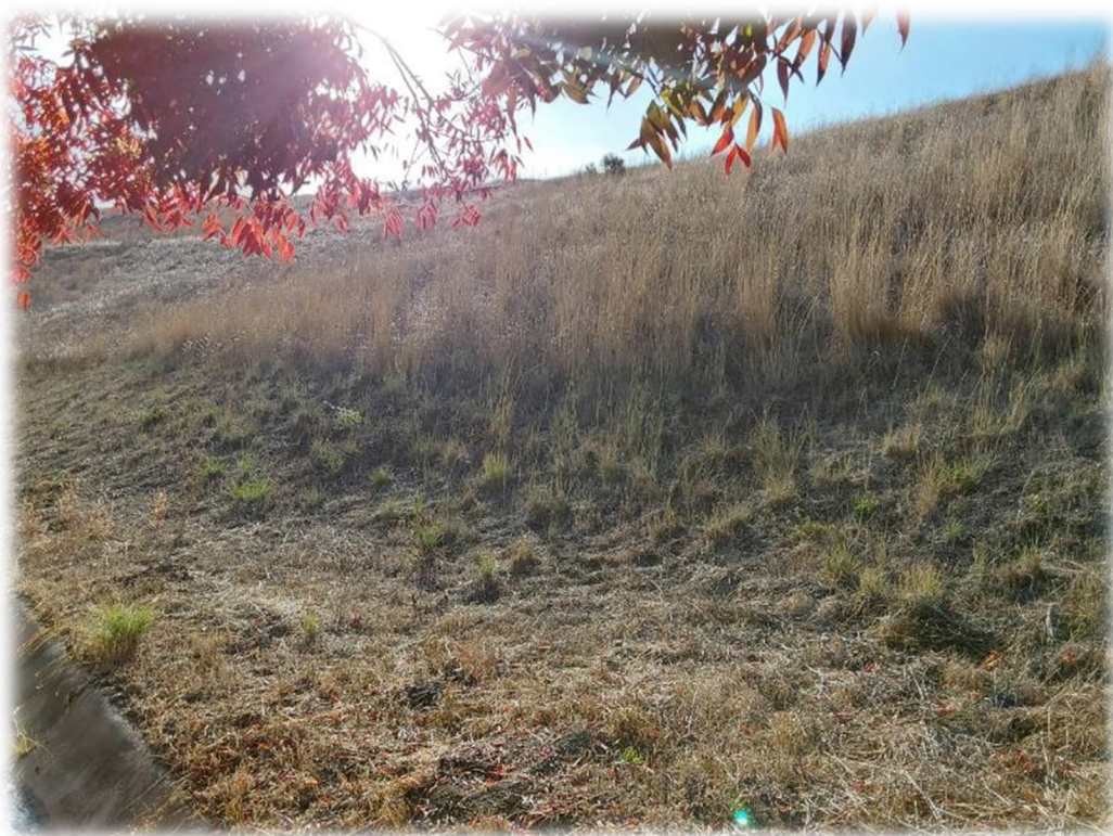
Photograph 22 – Slope creep behind 1116 Peacock Creek Drive.
