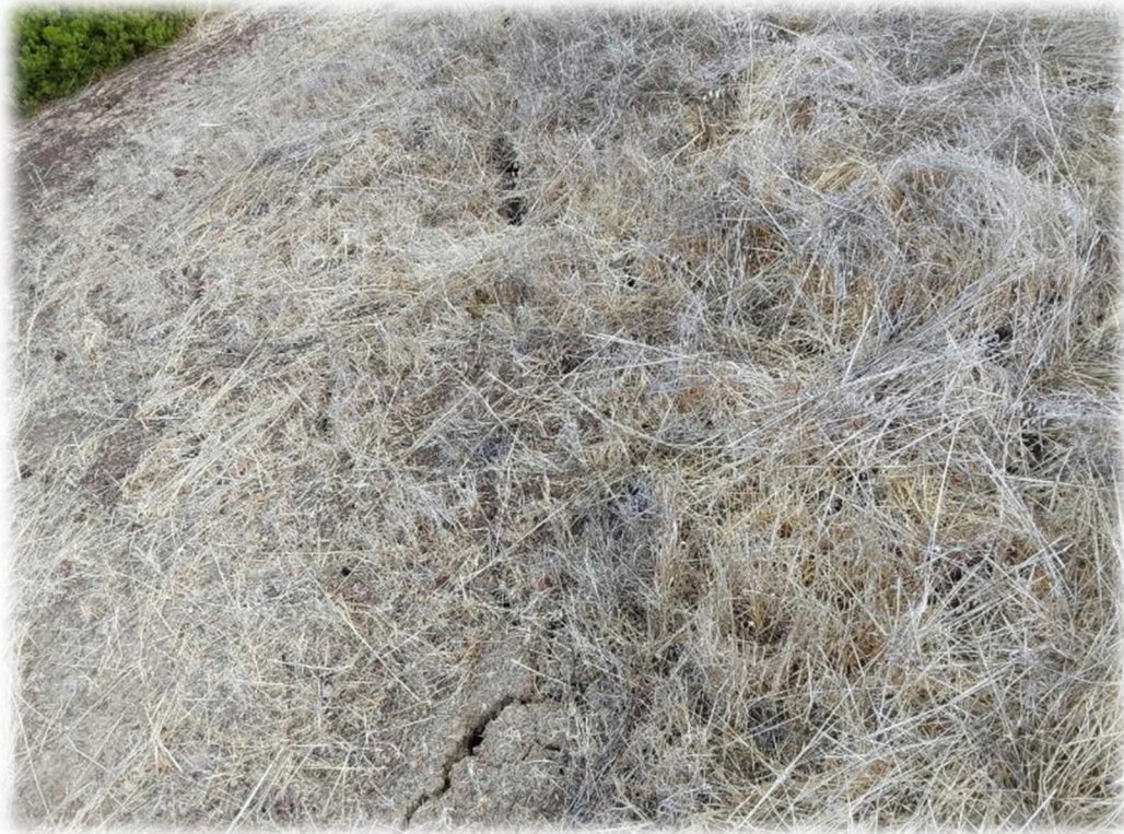
Photograph 17 – Possible slope creep/shrinkage cracks formed along the slope adjacent to/east of Peacock Creek Drive (approximately 40 feet from roadway).
