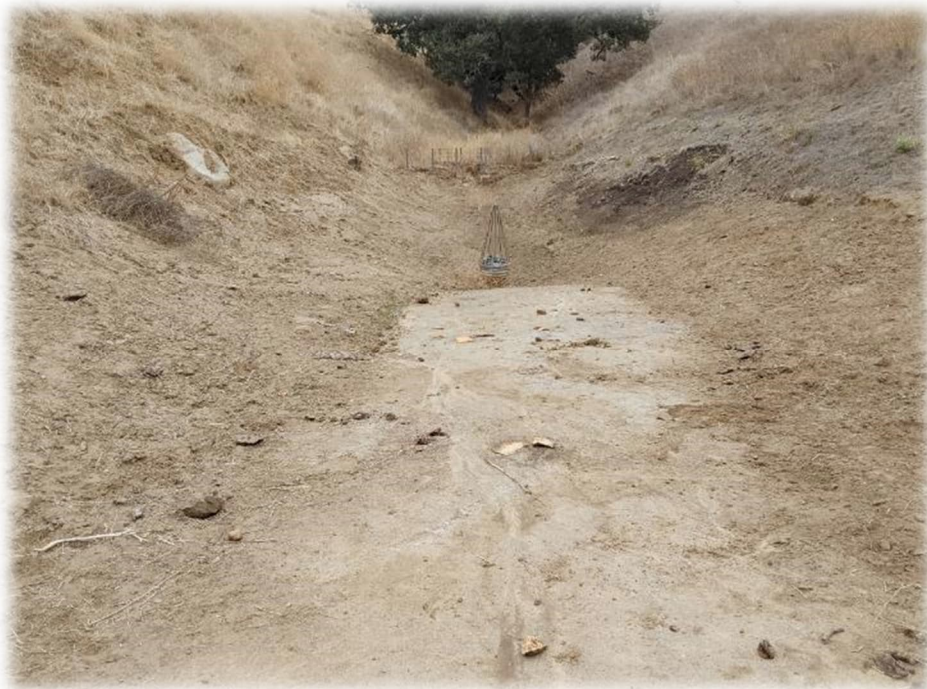
Photograph 4 – Current condition of containment basin northeast of Windmill Canyon Drive. The vertical corrugated metal pipe (CMP) riser contains some soil within it that has accumulated over time. Cleaning of this pipe should be performed.
