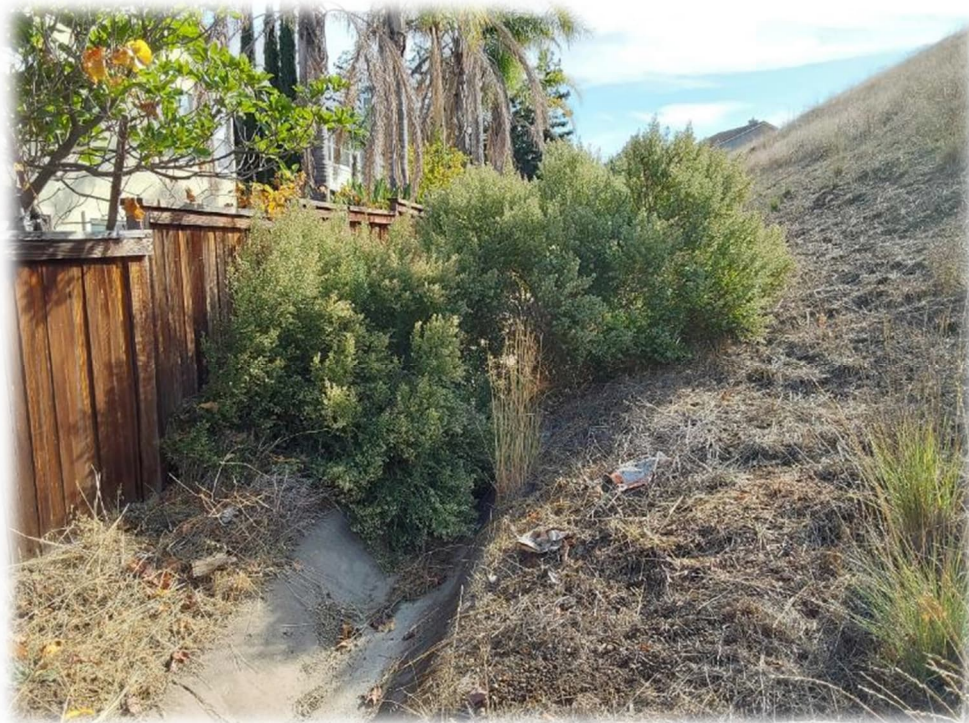
Photograph 26 – Vegetation within V-ditch present just east of Photograph 25 nearly blocks the V-Ditch. Vegetation should be removed from the V-ditch.
