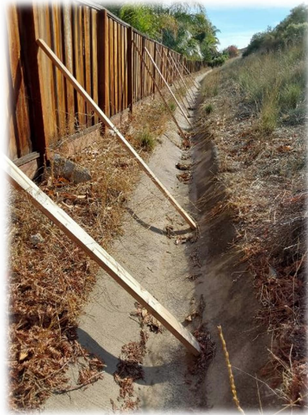
Photograph 25 – Resident has added fence supports within v-ditch near 1146/1148 Peacock Drive.
