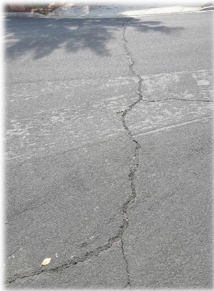
Photograph 33 – Cracks had been filled by City crew within pavement along Torrey Pines as of 11-17-2023.
