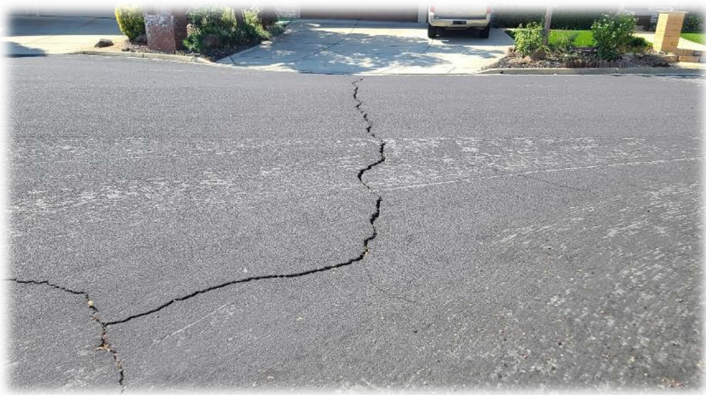
Photograph 32 – Numerous cracks observed within pavement along Torrey Pines on 8-31-2023. No cracks observed by residents within homes. No cracks observed along slope east of Torrey Pines.
