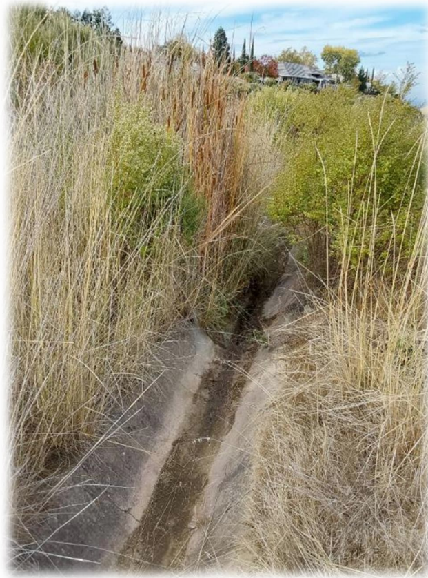
Photograph 34 – Similar conditions observed as noted in March 9, 2023 letter, Photo Q: moist ground and seepage from the slope.
