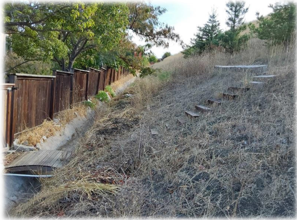
Photograph 23 – Similar conditions as noted in March 9, 2023 letter, Photo S, behind 1122 Peacock Creek Drive: Resident has planted trees and built a short keystone-type retaining wall uphill from the V-ditch.
