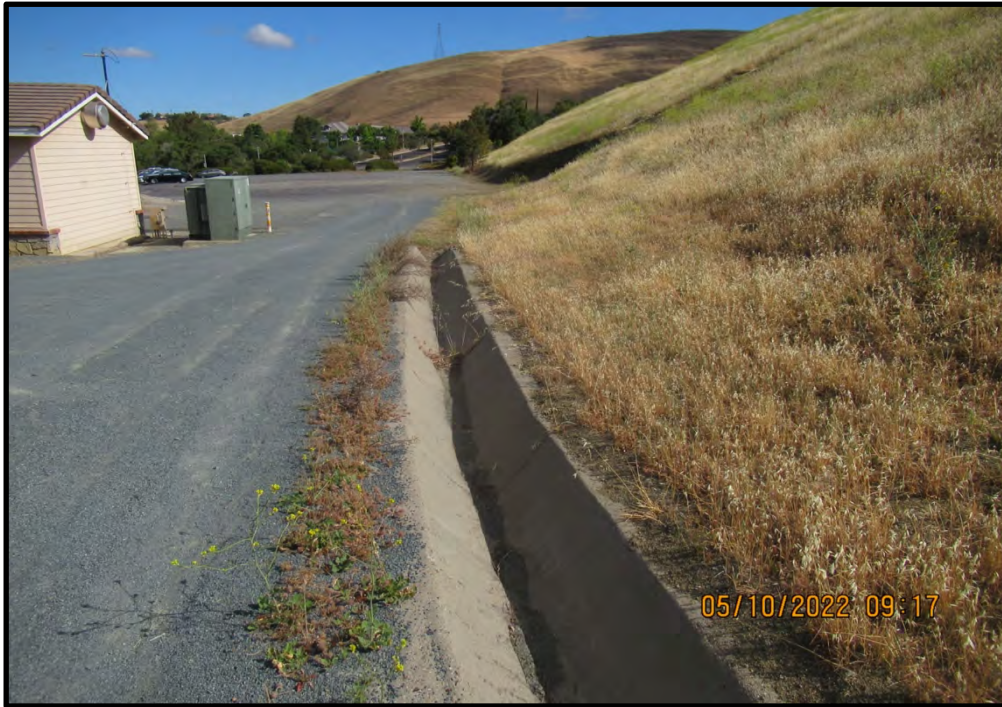
South part of the site, looking north from the south edge of the site; 05/10/22.
