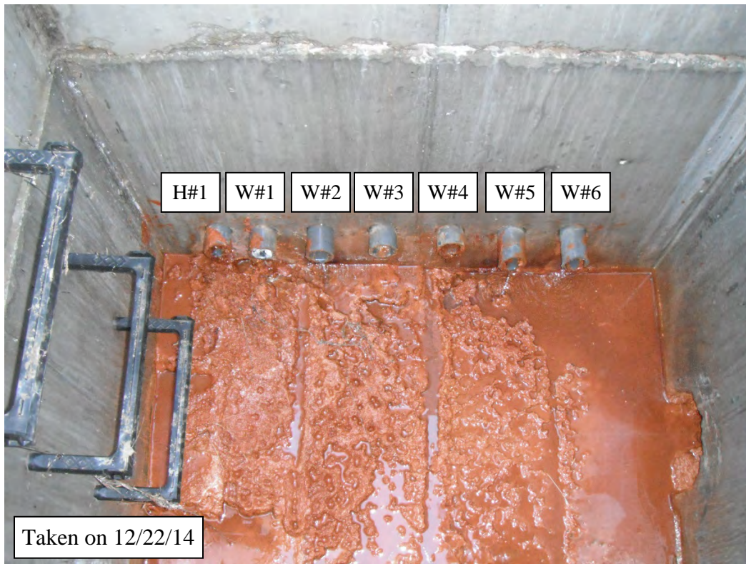
Figure 2, Photograph of Outlet Pipes
